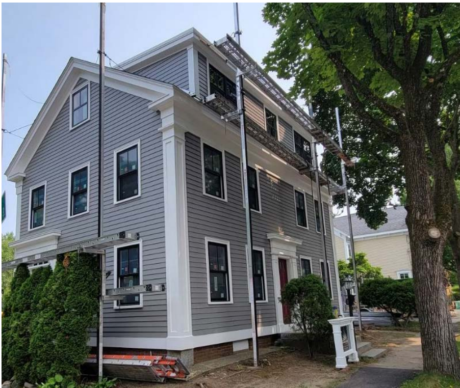
A process shot of a deep-energy retrofit of a historic house in Newburyport.
